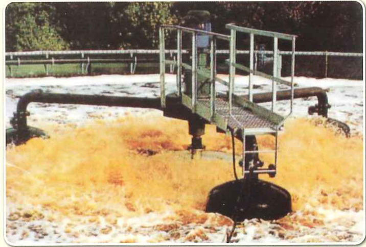
Floating Surface Aerator
