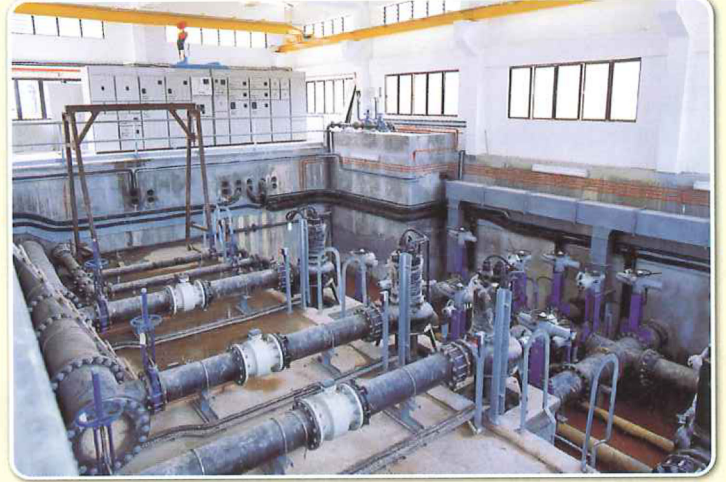
Sewage Pumping Station
