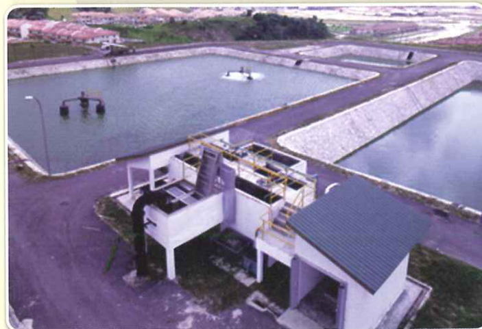
Aerated Lagoon In Operation
